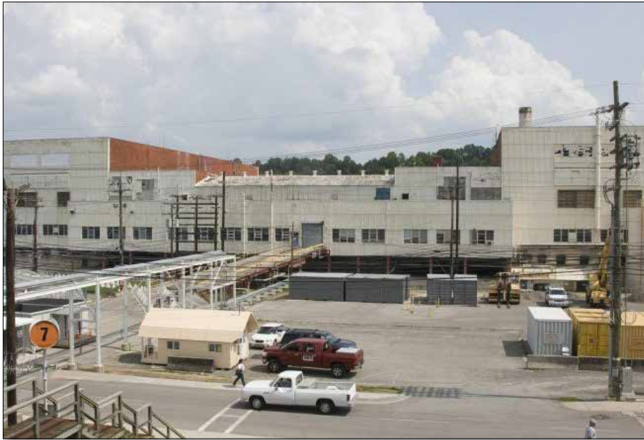
A view of the Alpha-4 facility at the Y-12 National Security Complex. Workers are in the early stages of removing all utility sources to the building prior to demolition.
