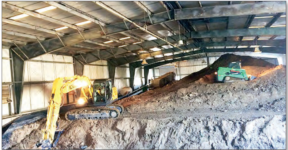
Equipment removes more than 4,000 cubic yards of soil for disposal from an Oak Ridge Site facility where it had been stored since 1989.
