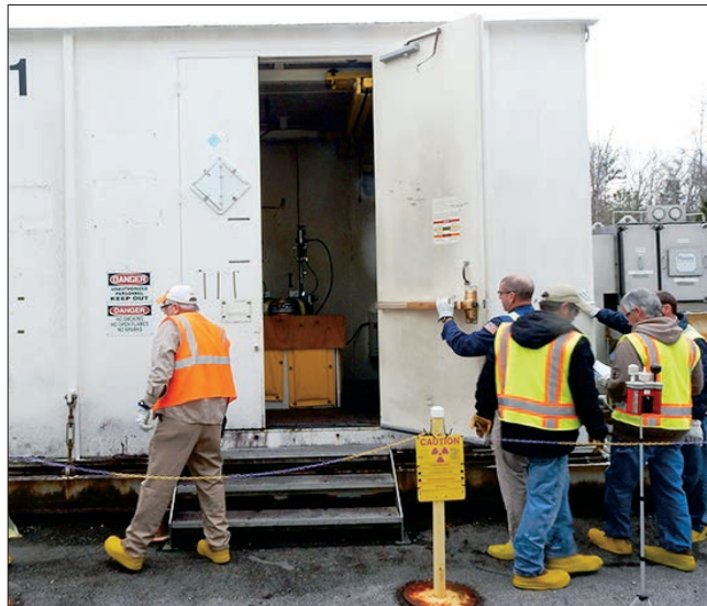
Workers prepare to install vents in drums of old TRU in a closed, explosion-proof, high-efficiency particulate air-ventilated unit.
