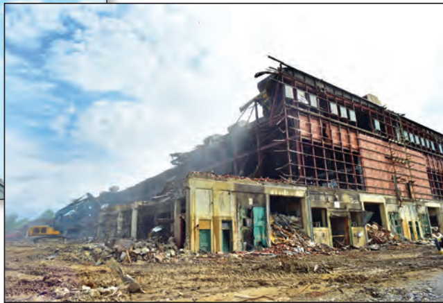
Left, demolition began at building K-27 on February 8, 2016. Right, progress on K-27 in May 2016 (photo by Lynn Freeny).
