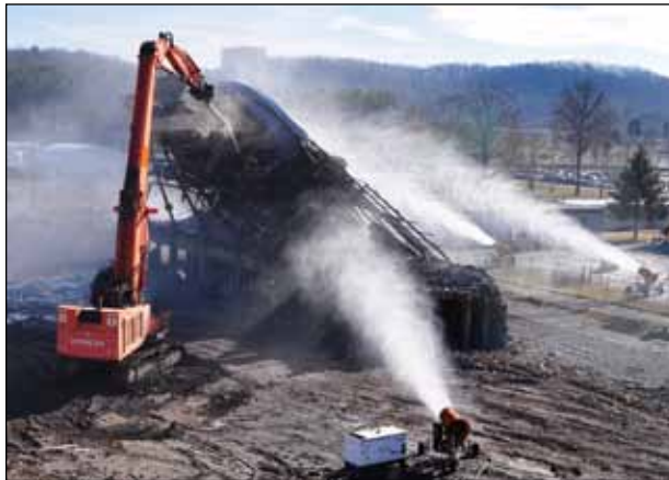
The last standing section of the K-25 Building is pulled to the ground signalling the final demolition of the old building.
