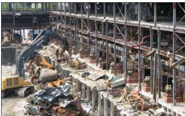
Demolition of the K-25 building at ETTP is proceeding steadily north along the east wing of the building.
