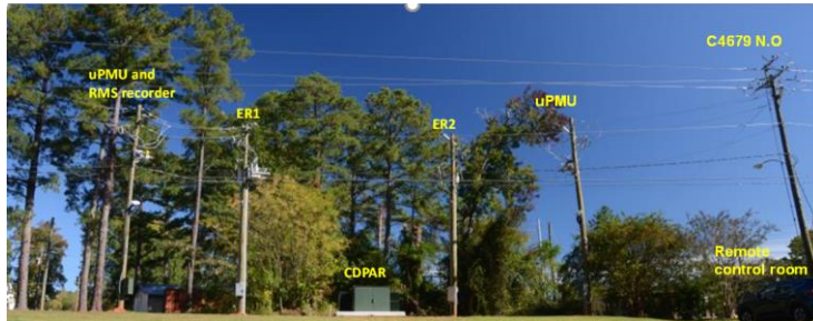
13 kV 1 MW Power Router Field Demo
