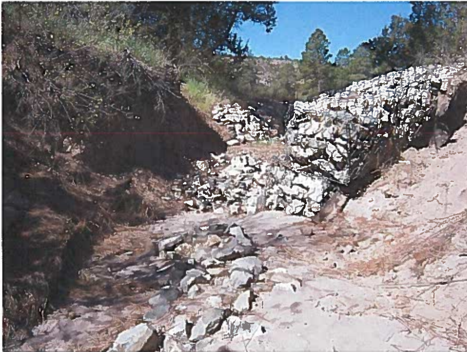
Photograph 4. The channel below dissipation structure will be restructured and the gabion removed.
