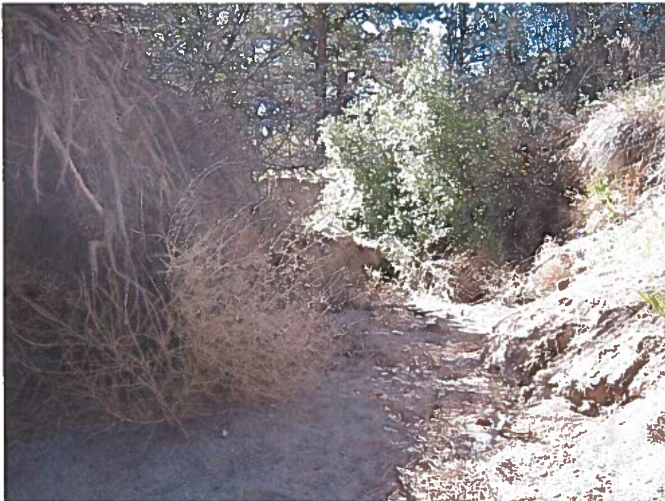
Photograph 5. View of channel degradation and erosion in the sharp bend.
