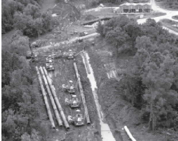
1978 construction of a DOE crude oil pipeline in bottomland hardwoods/wetlands near the SPR Bayou Choctaw Facility (DOE file photo).
