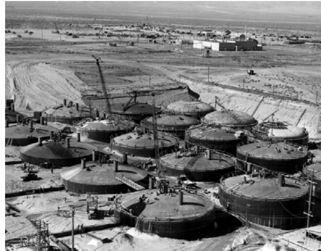
The Hanford Site's single-shell underground storage tank system was built from 1943–1964. The Draft EIS analyzes the potential environmental impacts of closure of Hanford's 149 single-shell tanks.
