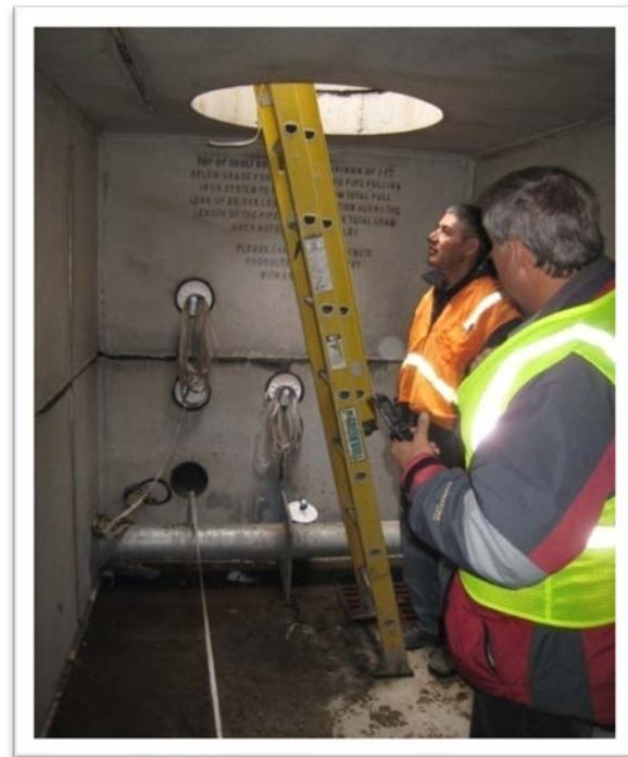
Interior of a vault, before cable installation, for 230-kV transmission line in Denver
