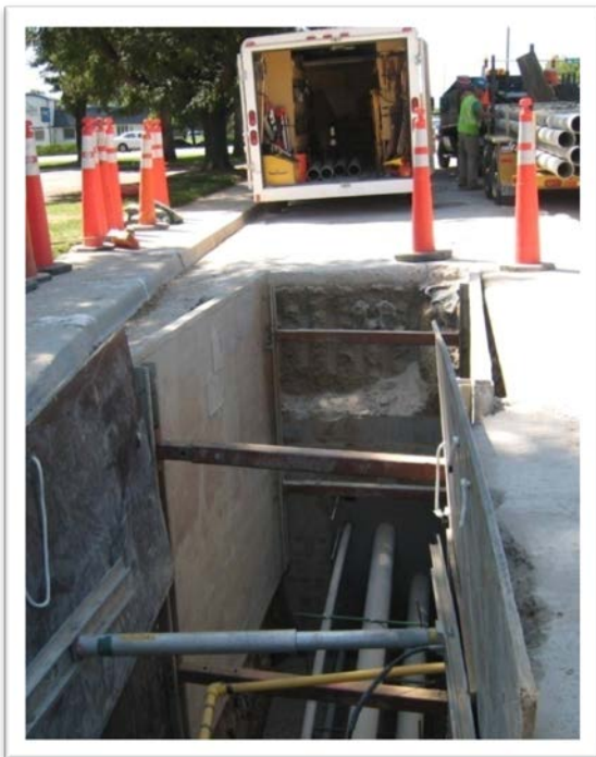
Exposed sections of conduits, duct bank, and backfill constructed for 230-kV in Longmont
