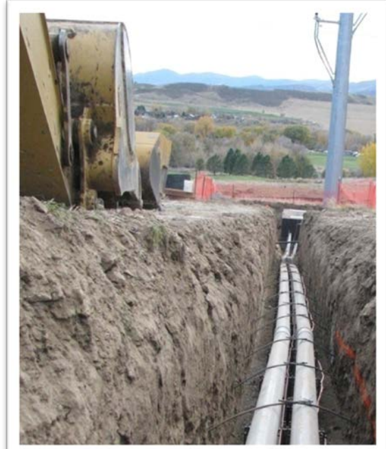
115-kV duct and termination structure in open space in Jefferson County, Colorado
