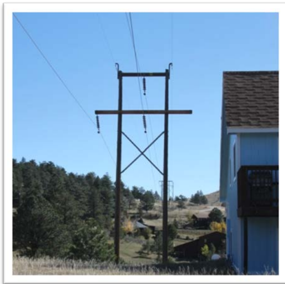
Photograph of E-LS through the Newell Lake View subdivision where a number of buildings are immediately adjacent to a 20-foot ROW.
