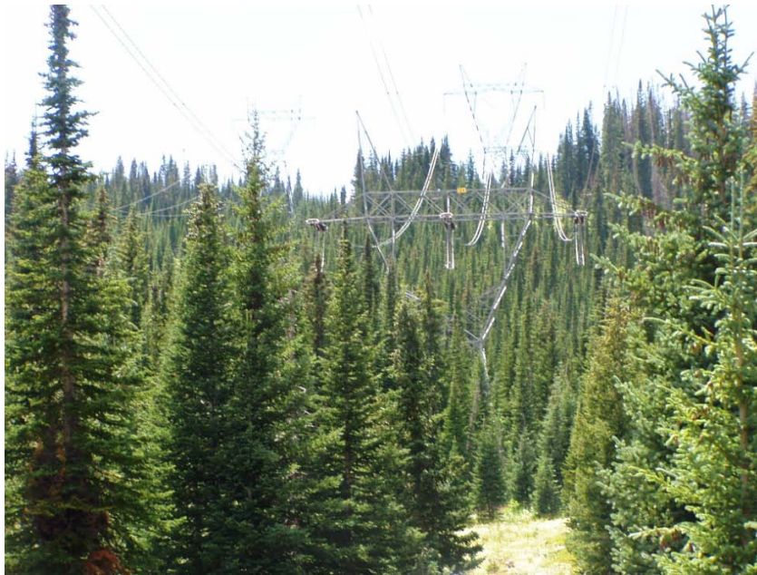
Photo 2-11. This ROW condition is not acceptable because of the risk the trees pose to the transmission line conductors, and poor access for maintenance.
