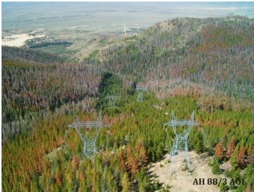
Photo 2-6. The lodgepole pine in the ROW is rapidly re-growing and would need to be treated and maintained.
