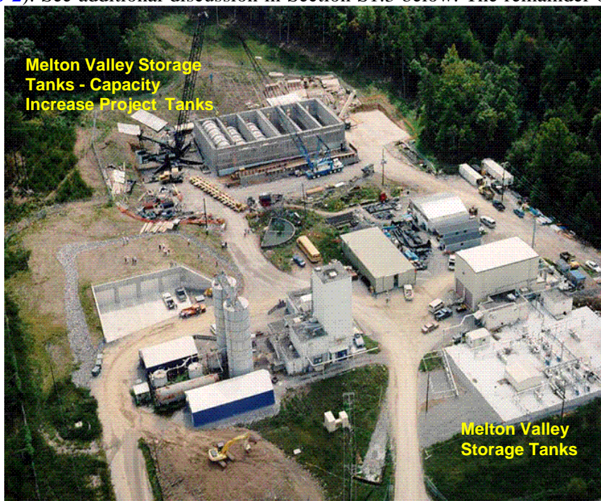
Figure S-2. Aerial view of the Melton Valley Storage Tanks–Capacity Increase Project during installation of the six 100,000-gallon tanks, which are located south of the eight 50,000-gallon Melton Valley Storage Tanks.
