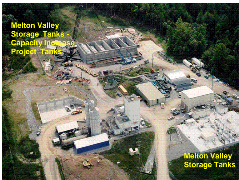
Figure 1-2. Aerial view of the Melton Valley Storage Tanks–Capacity Increase Project during installation of the six 100,000-gallon tanks located south of the Melton Valley Storage Tanks.
