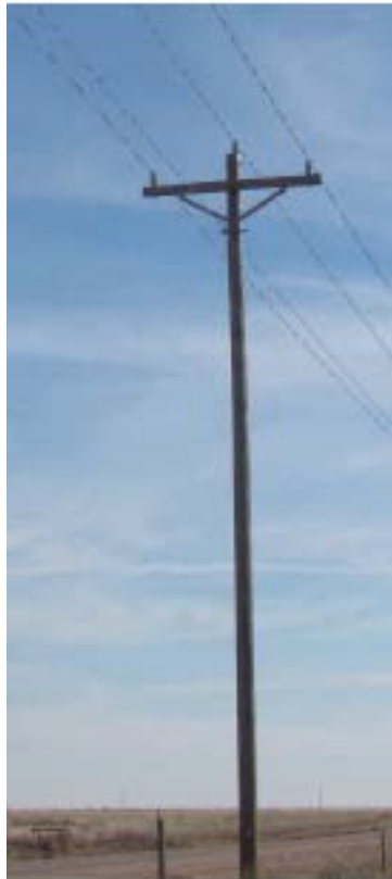
Figure 12. Typical Distribution Line Pole.
