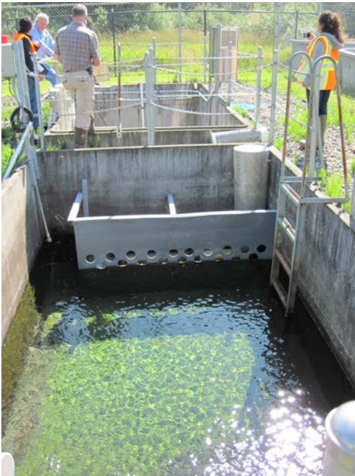
Photograph 2 – The settling basin and UV treatment system for the Burley Creek Hatchery (view looking east).
