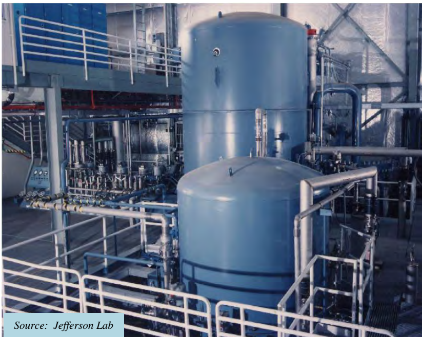
Figure 2-5 Typical Cryogenic Plant Equipment (Cold Box)
