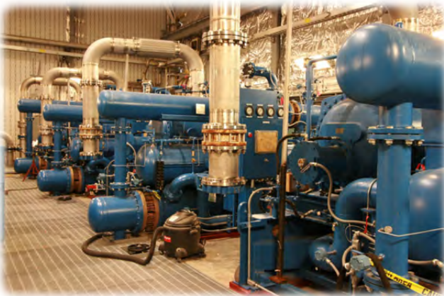
Figure 3-10 Cryogenic Plant Compressor Room
