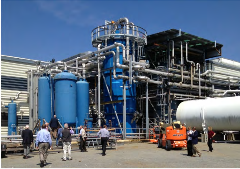
Figure 3-9 Cryogenic Plant at Thomas Jefferson National Accelerator Facility
