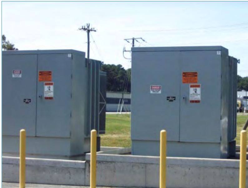
Figure 2-6 Typical Cryogenic Plant Transformers
