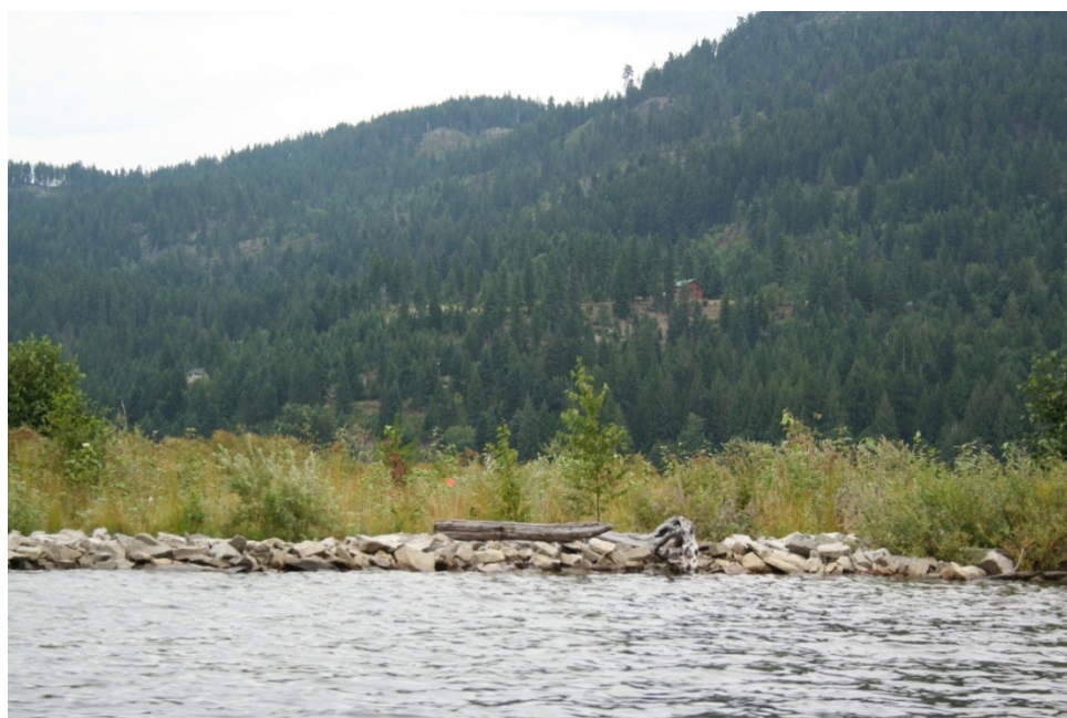
Figure B-8: Example of riprapped shoreline protection with woody debris and managed vegetation; Pack River nearly 5 years after establishment.
