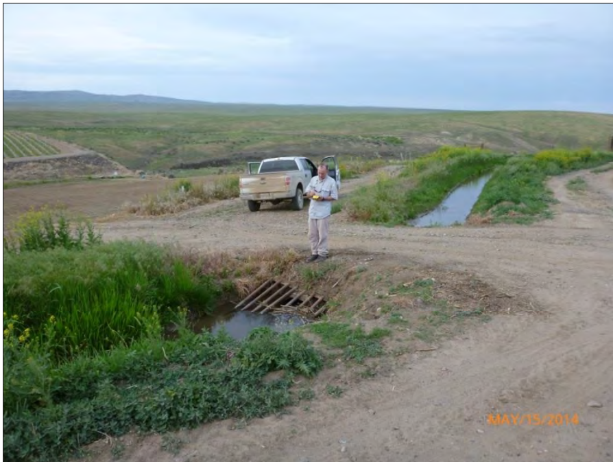
Figure 3.10-5. Photograph shows an existing culvert in an irrigation ditch between Structures 23/7 and 24/1 in Line Mile 23 that would be replaced. This ditch has been identified as a perennial waterway. (Source: Tetra Tech 2014d)
