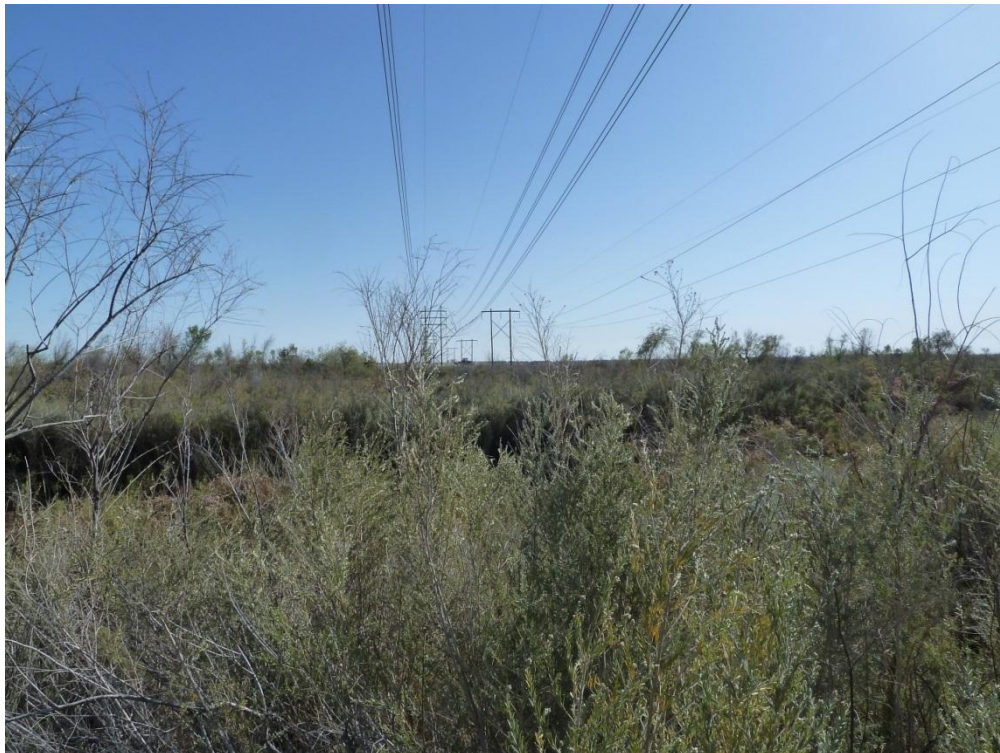
Photo 2 – View looking south at structures 2-6 and the span over the Gila River.
