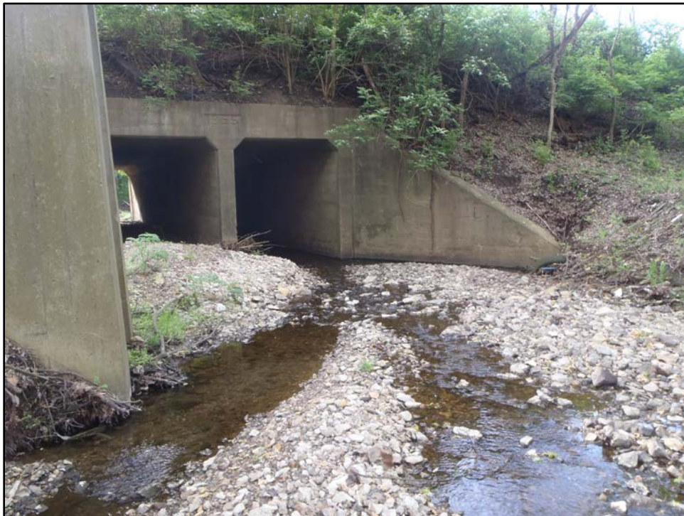
Photograph C-2: View of intermittent stream S-1, facing east. A support structure for the overhead sewer line is visible in the left side of the photograph.
