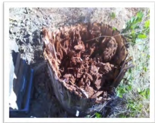
Figure 1-2. Decayed Wood Pole
