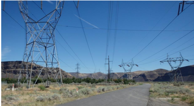
Photo 3.10-2. Representative density of transmission lines in the project area; the transmission lines above parallel Palisades Road which is located near the southern end of the East Route
