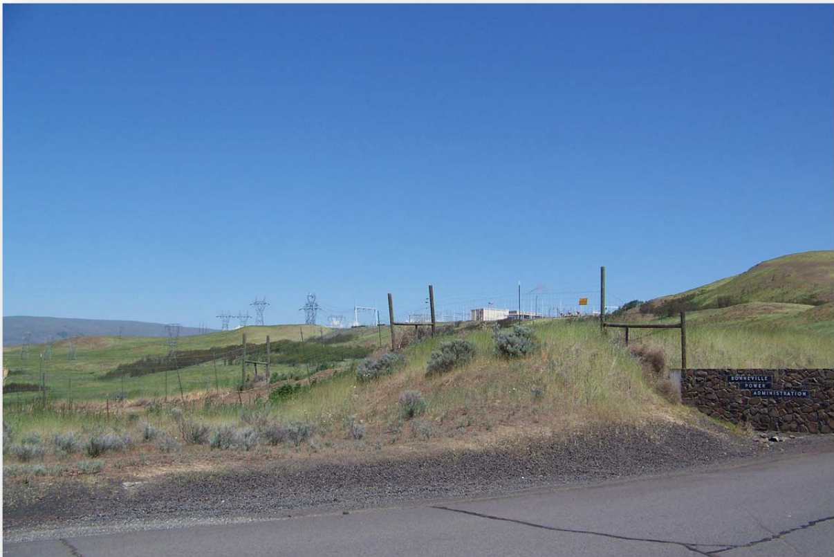
Figure 3.9-1: Celilo Converter Station South of The Dalles on US 197
