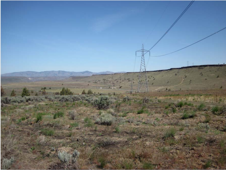
Figure 3.9-2: Transmission Line Crossing of US 97 at Tower 61/1
