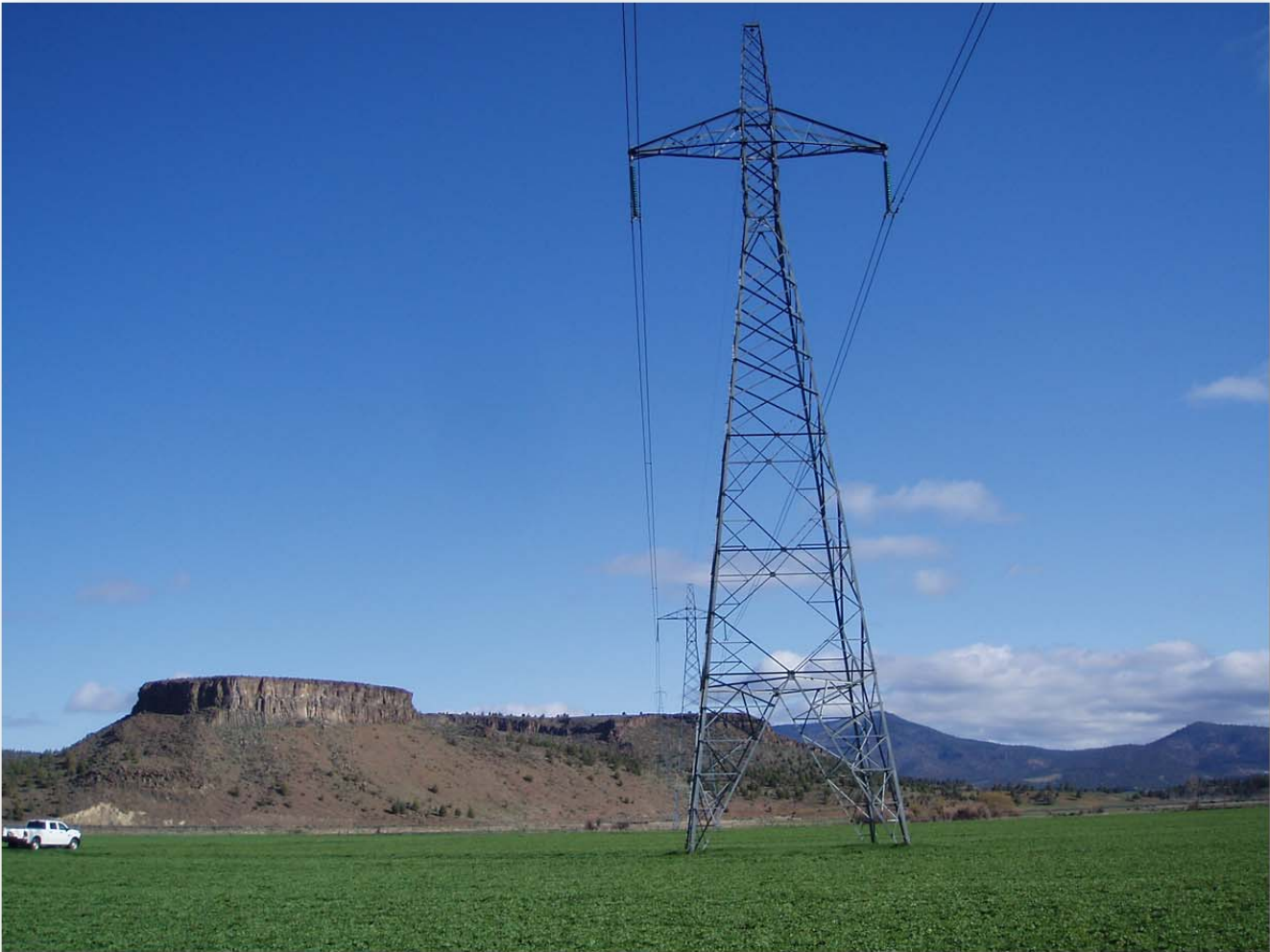
Figure 2.1-3: Existing PDCI Line Irrigated Agricultural Land South of the Crooked River (Tower 91/2 looking south)
