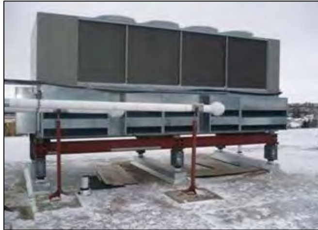
Figure C-2. Photo of HVAC rooftop unit on commercial building roof.
