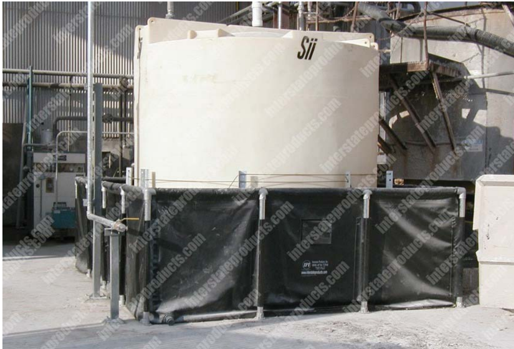
Figure 3.5: Example commercial secondary containment system which would be attached to the interior side of the drywall walls of the IPND structure inside the existing MINOS Service Building.
