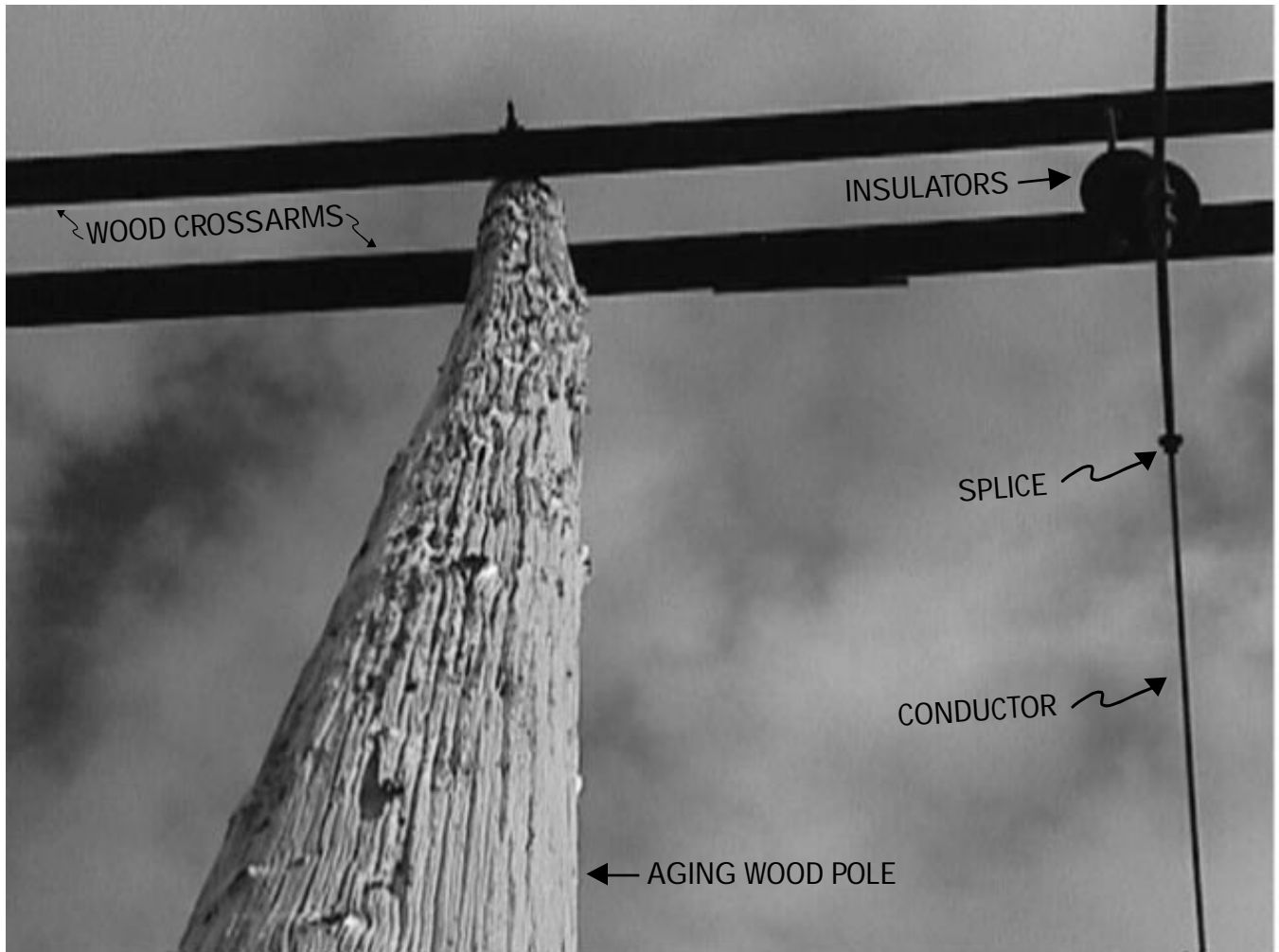
EXISTING POLE – REEDSPORT-FAIRVIEW LINE
