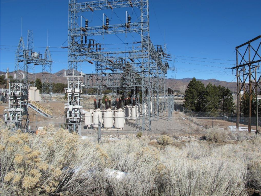
South Side of Existing Substation
