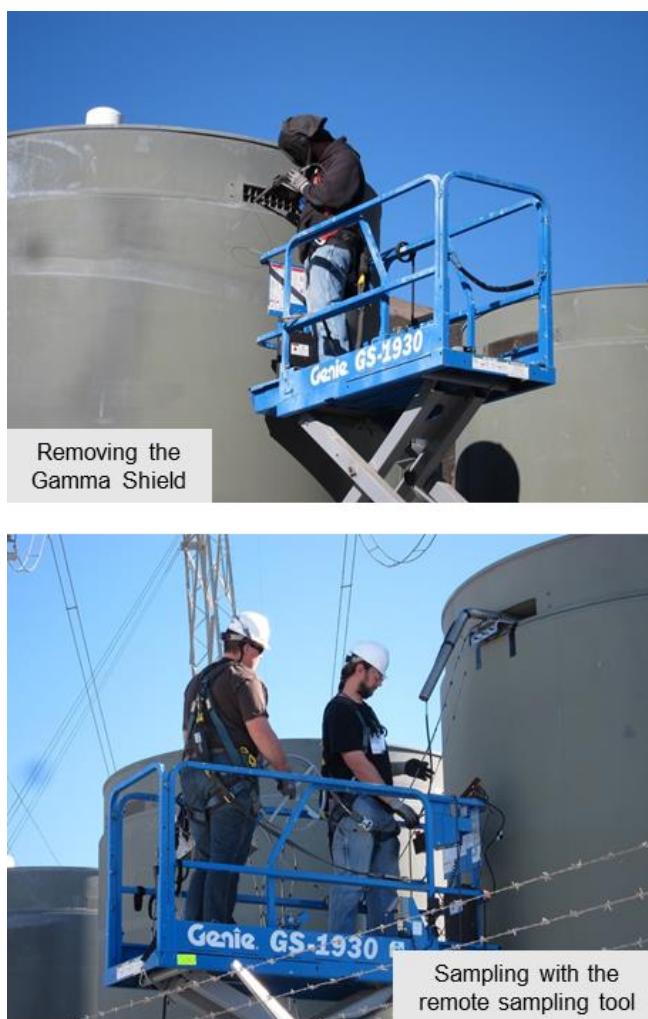
Figure 2. Sampling dust from the surface of interim storage canisters within their overpacks.
