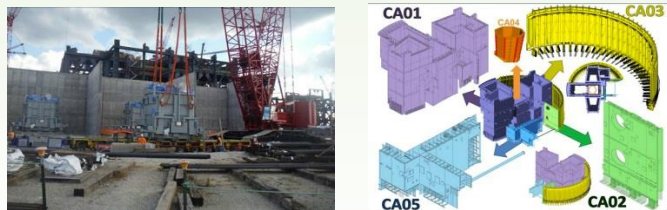
Unit 2 transformer is set in place; schematic of containment structural modules (Courtesy of SCANA)
