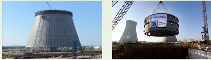
Progress on Unit 4 cooling tower; CV ring lowered into place (Courtesy of Georgia Power/Southern Company)
