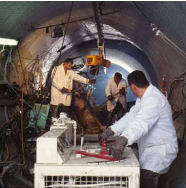
Swiss scientists investigate the influence of groundwater on radioactive substances in the rock.
