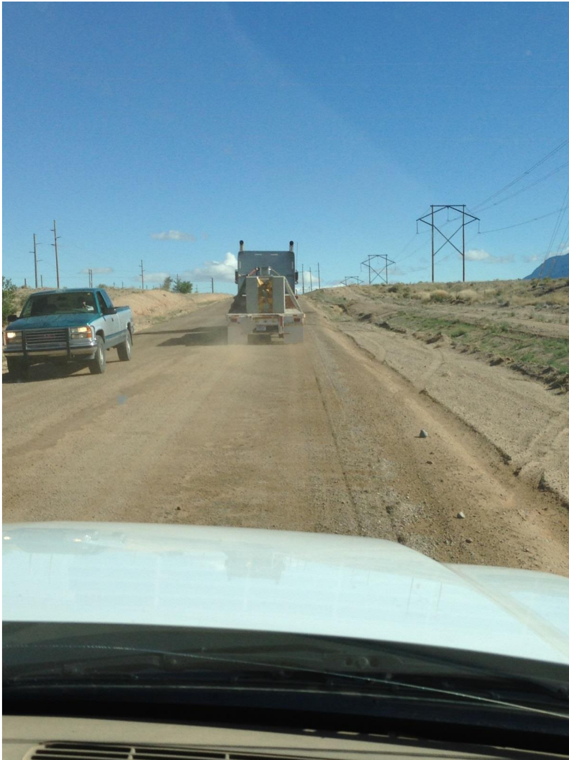
Figure 4.8 Poleline Road approaching Eubank Contractors' Gate, Segment 1. This potholed, dirt/gravel portion of the truck route resulted in the highest measured rod strains.
