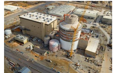
Vogtle Unit 3 (Courtesy of Georgia Power/ Southern Company, April 2021)
