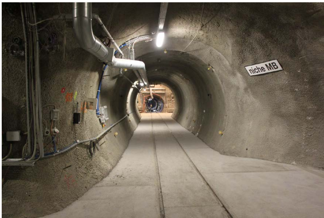
Figure 3.1-7 View from the FE gallery into the heater tunnel during final installation (Bossart 2014a).
