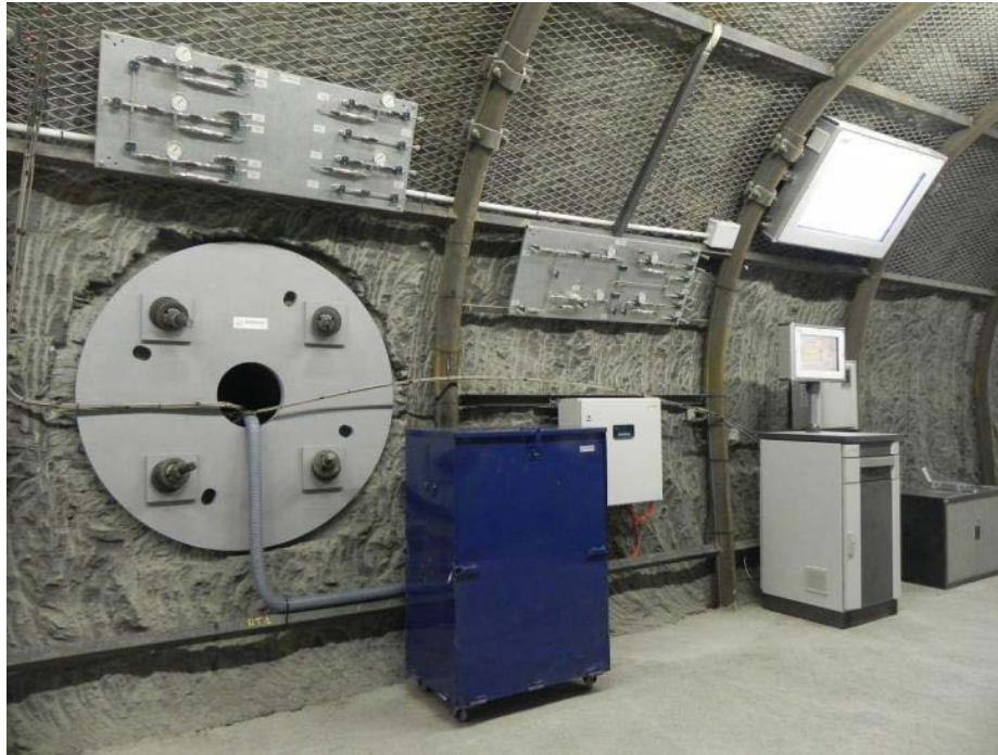
Figure 3.2-3 SEALEX Experiment at the Tournemire URL: View of mini-tunnel from gallery after seal emplacement (Barnichon 2011).
