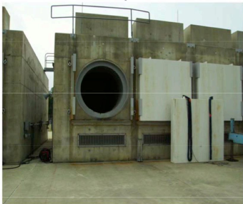
Figure 3. NUHOMS horizontal storage module, at the Calvert Cliffs ISFSI, with doorway open for storage container insertion. The air inlet vent is below the door (Figure 1.2, Suffield et al., 2012).
