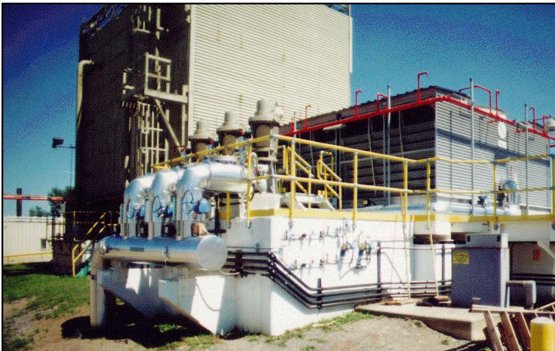
Figure 3-40. The New Cooling Tower. (The cooling tower will be removed, except for its concrete basin, before Phase 1 decommissioning activities begin.)
