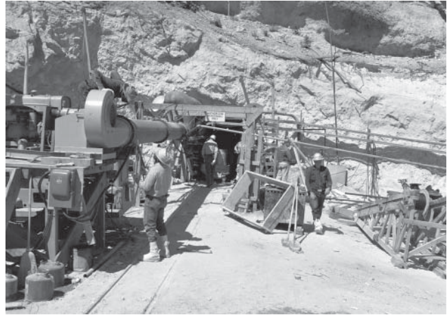
Mouth of the Rainier tunnel prior to the shot while construction was still in progress. Large pipe at left is part of the blower system to supply fresh air to workmen in the tunnel. Source: DOE, NNSA-Nevada Site Office.
