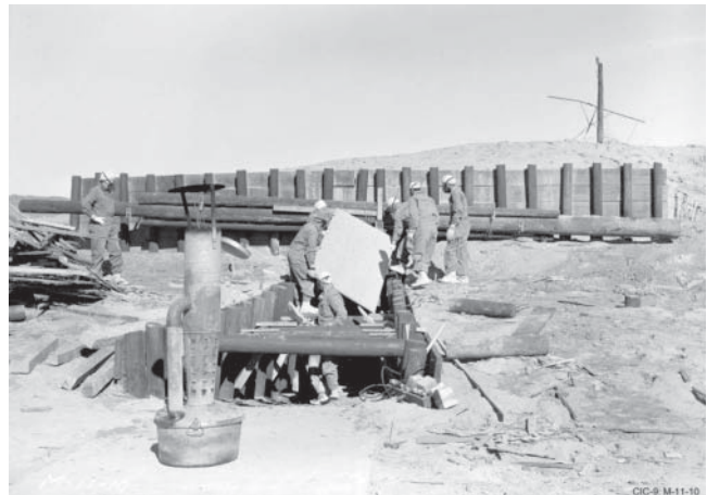
Workers repairing the blockhouse on January 31, 1951, following Baker. Note the protective masks and foot coverings. Source: Los Alamos National Laboratory.
