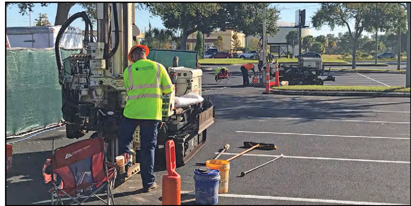
Direct-push rigs used for the bioinjection process at the Pinellas County site.
