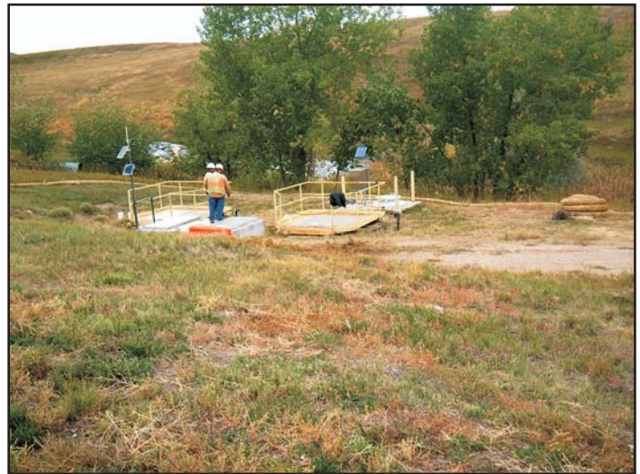
The East Trenches Plume Treatment System prior to the media replacement project.
