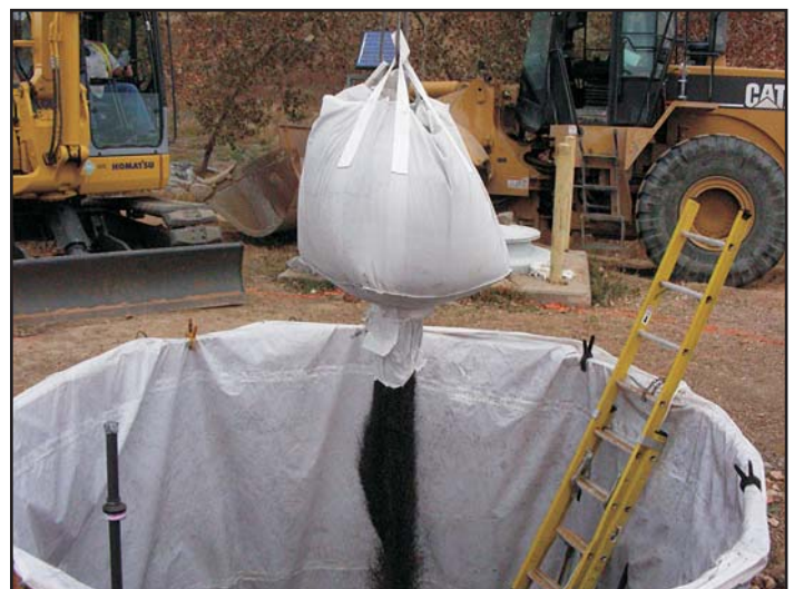
New ZVI media is placed into one of the treatment cells. The new liner in the cell is also visible.
