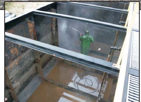
Photos top to bottom: SSTP being assembled in 2005; sludge-dewatering equipment; dewatered sludge after removal from SSTP; pressure washing SSTP tank.
