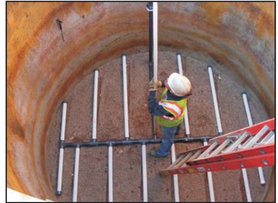
A contractor installs the plumbing that distributes the water to be treated in the cell.
