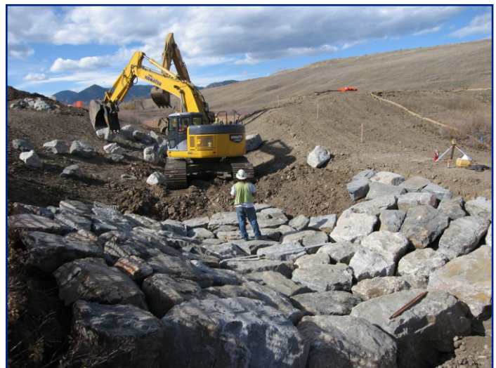
An excavator places large stone riprap for erosion control prior to installing the stoplog structure during the dam breaching project.
