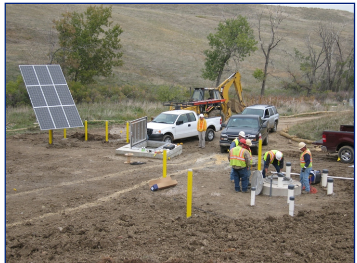
An LM crew works on the solar powered pump system at the Solar Ponds Plume Treatment System.
