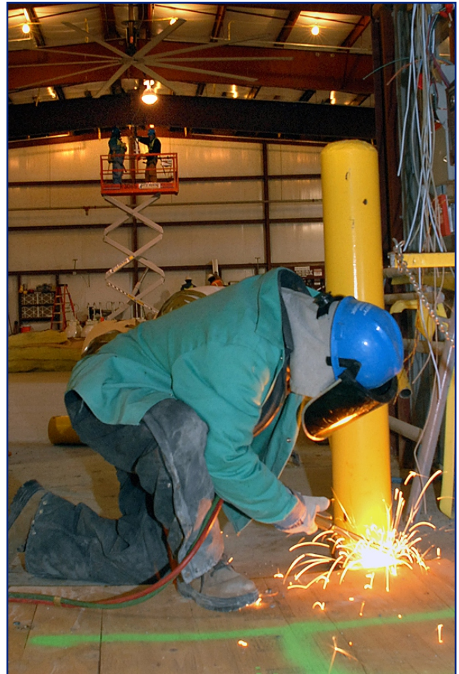
Work proceeding on the proposed Fernald Preserve Visitors Center. Recycle and reuse of materials from the building is a high priority.
