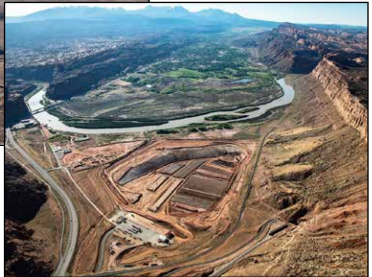
The tailings pile at the former Atlas Uranium Mill site in Moab, Utah, after the start of removal and relocation to the Crescent Junction site (2018).
