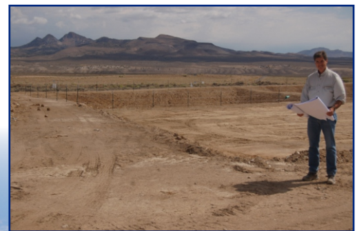
DOE Site Manager Mark Kautsky inspects the completed well pads at the MV-5 drill pad, Central Nevada Test Area.
