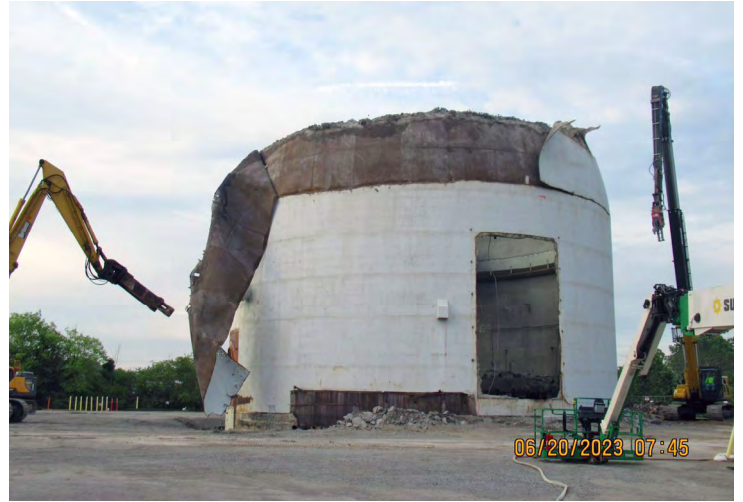
Phase 4 required elevated torch cutting the dome’s steel skin, then “peeling” it away before demolishing the concrete reactor building from the top down.
