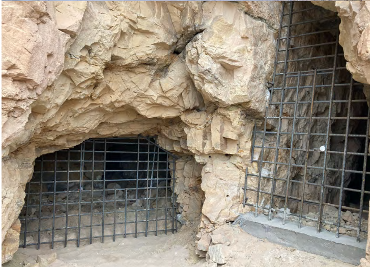
Adits at the Mucho Claims Mine, located southwest of Green River, Utah, before and after safeguarding (BLM-administered land).
