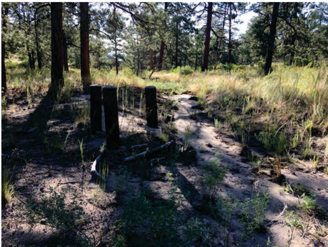
Photo 6. Soil Erosion Occurring at Base of Protective Bollards
