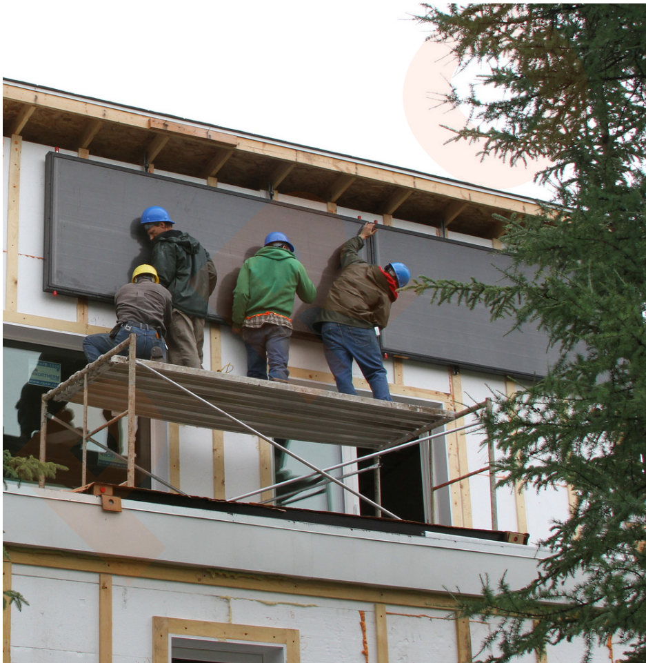
Four workers install solar photovoltaic panels on a house in Alaska. Photo from Cold Climate Housing Research Center
