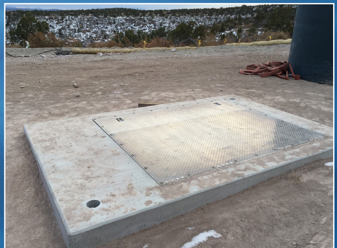
The closed vault at injection well CrIN-5 helps reduce the project's footprint.
