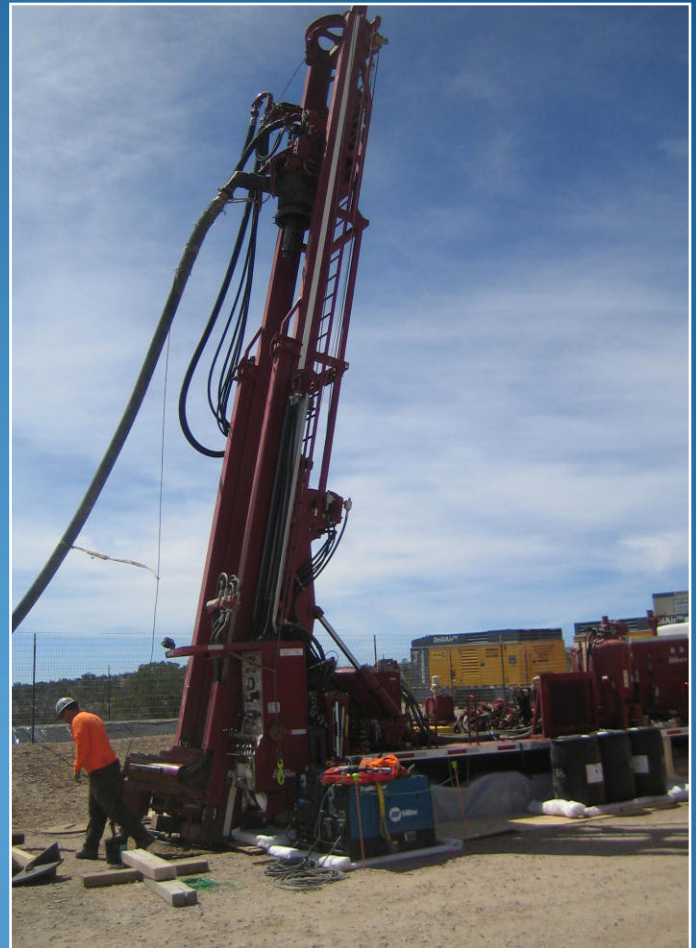
An angled drill was used to install the injection well CrIN-4 and avoid sensitive areas.
