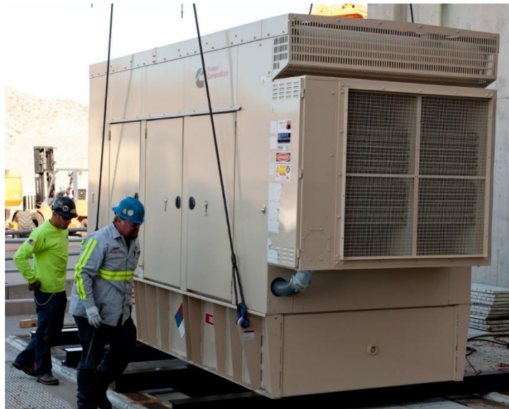
Figure 21. Workers installing a 500 kW emergency generator at Davis Dam. Source: US Bureau of Reclamation, photograph # B351-300-20437
