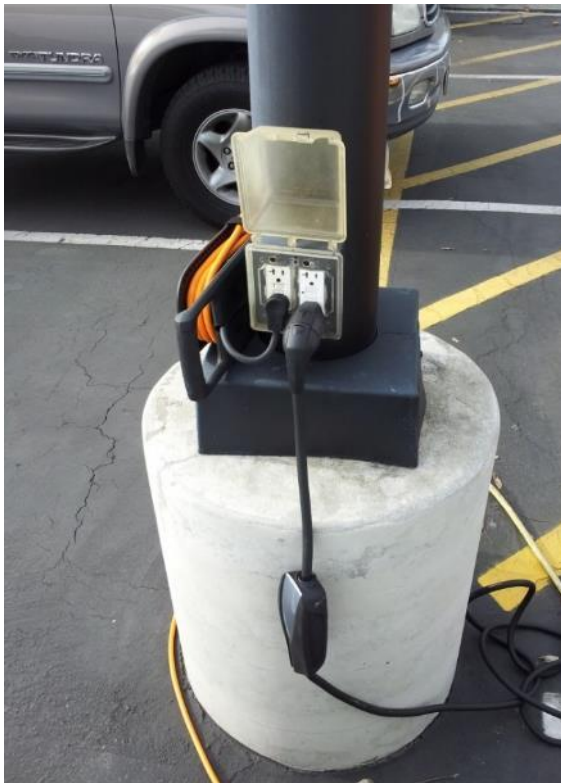
Photo 9. Level 1 charging receptacles can be installed on parking lot lamp posts. Photo from Idaho National Laboratory.
