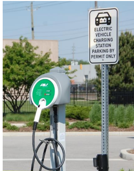
Photo 8. In 2010 Eli Lilly & Company installed several workplace charging stations at its two main campuses in Indianapolis, IN. Photo from Eli Lilly.
