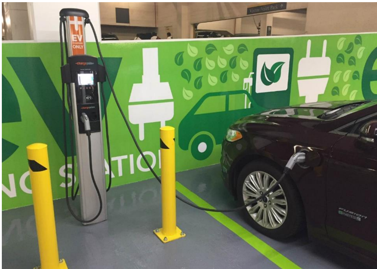
Photo 4. PEV charging stations within a downtown Los Angeles parking garage. Photo from Kendall Septon, NREL 37582.
