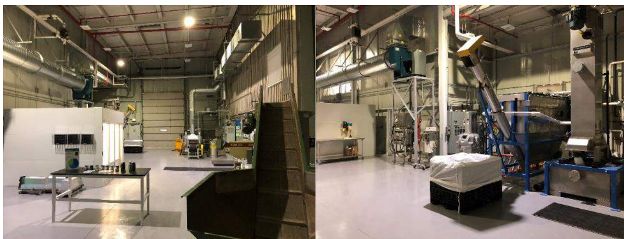
Figure I.4.C.2 ReCell Pilot Scale High-bay located at Argonne National Laboratory Building 369
