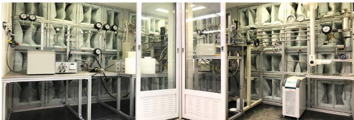
Figure I.2.G.1 Installed supercritical fluids system for processing battery cathode materials
